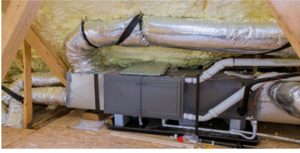
Typical air handler set-up with drain pan and condensate drain
